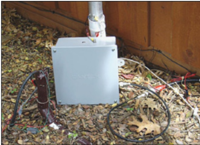
Figure 10 — The completed all band remotely controlled switching and impedance matching network mounted at the antenna base.
